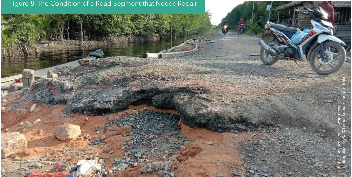
Figure 8. The Condition of a Road Segment that Needs Repair
