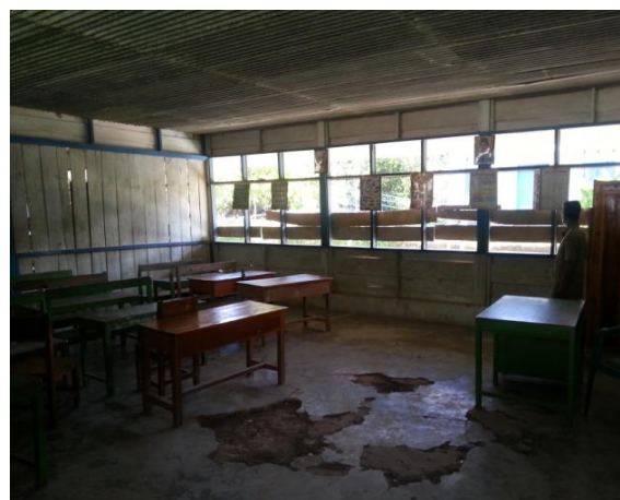
A poorly maintained classroom
